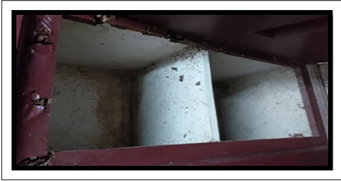
Figure 2. Damage to the wood.
